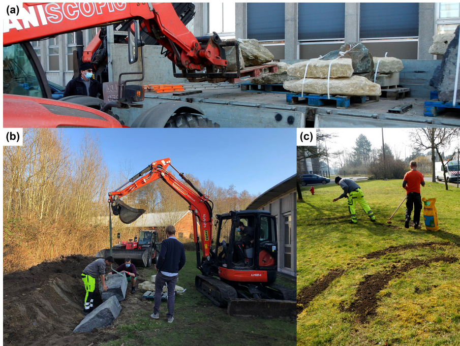
Figure 1. Installation of the Rock Garden at Ghent University. (a) Rocks were delivered in coordination with Monument NV and unloaded with the help of the Ghent University DGF. (b) Rocks were installed, under careful supervision, using both human and machine power. (c) After installation, green areas were reseeded with grass or wildflower seeds to ensure the full recovery of the green spaces.
